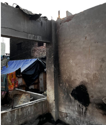
Fire damage in Korail, Dhaka, November 2025
